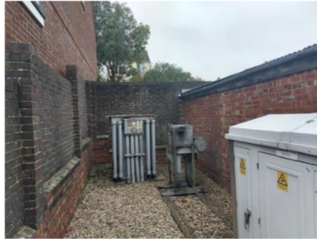
Fig 4.1 Photo of substation contents.
