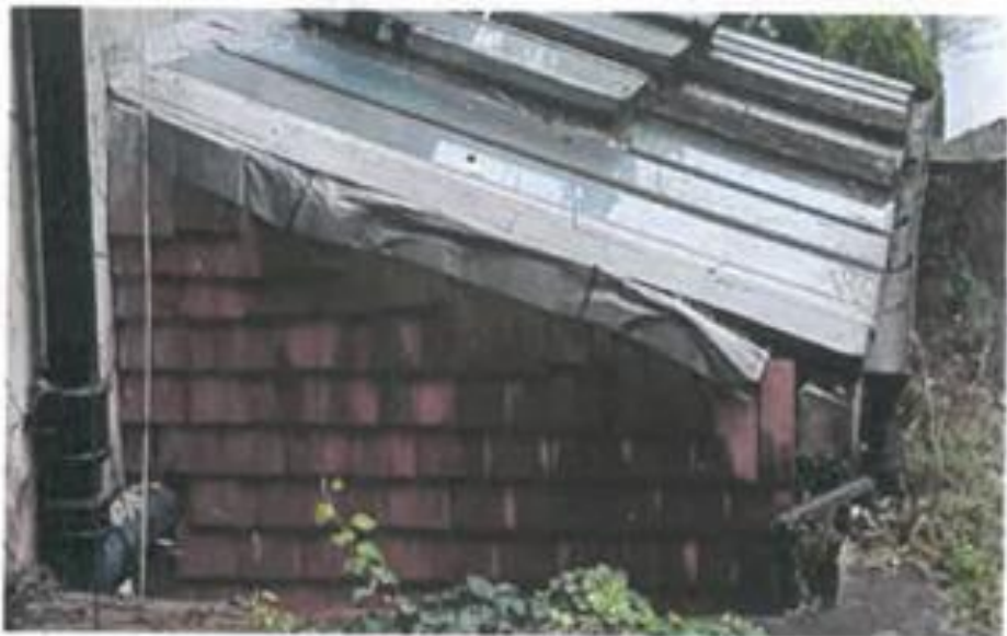
Tiles above the horizontal soil pipe connection through wall to be removed.
