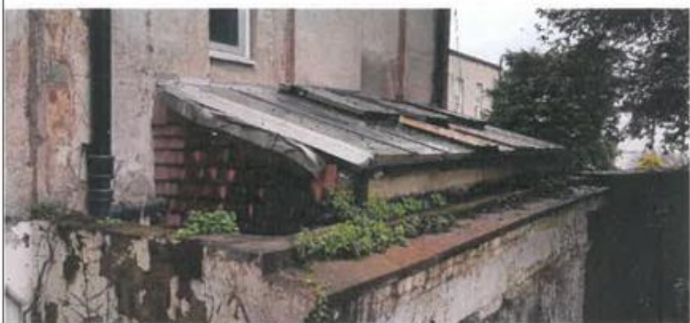
View from adjoining property. No work below stone coping to wall beneath
