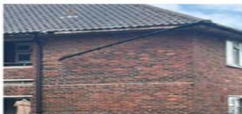
ABOVE: Guttering that has come away from downpipe and is hanging dangerously.
