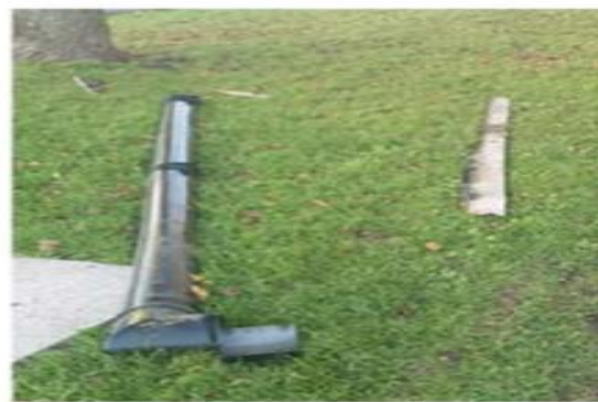
RIGHT: Length of guttering that fell away from The Lindens.
