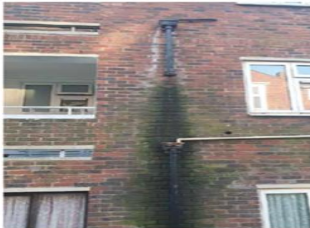
LEFT: The Lindens, showing damage caused by missing length of downpipe.
