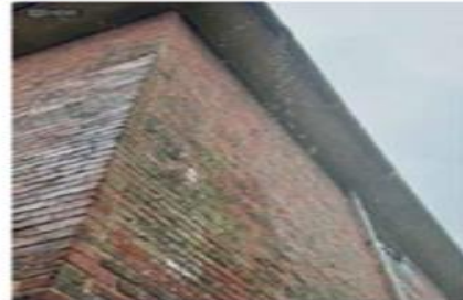
BELOW: The Cedars, taken during rainfall, showing overflow due to blocked gutter.
