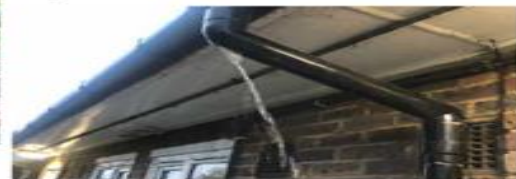
BELOW: Hollybank – overflowing gutter which was fitted only in 2017 as part of major works.
