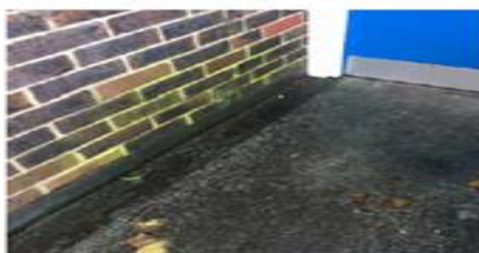
BELOW: Hollybank – mildew caused by lack of repairs to guttering. The guttering was only replaced in 2017 as part of major works.
