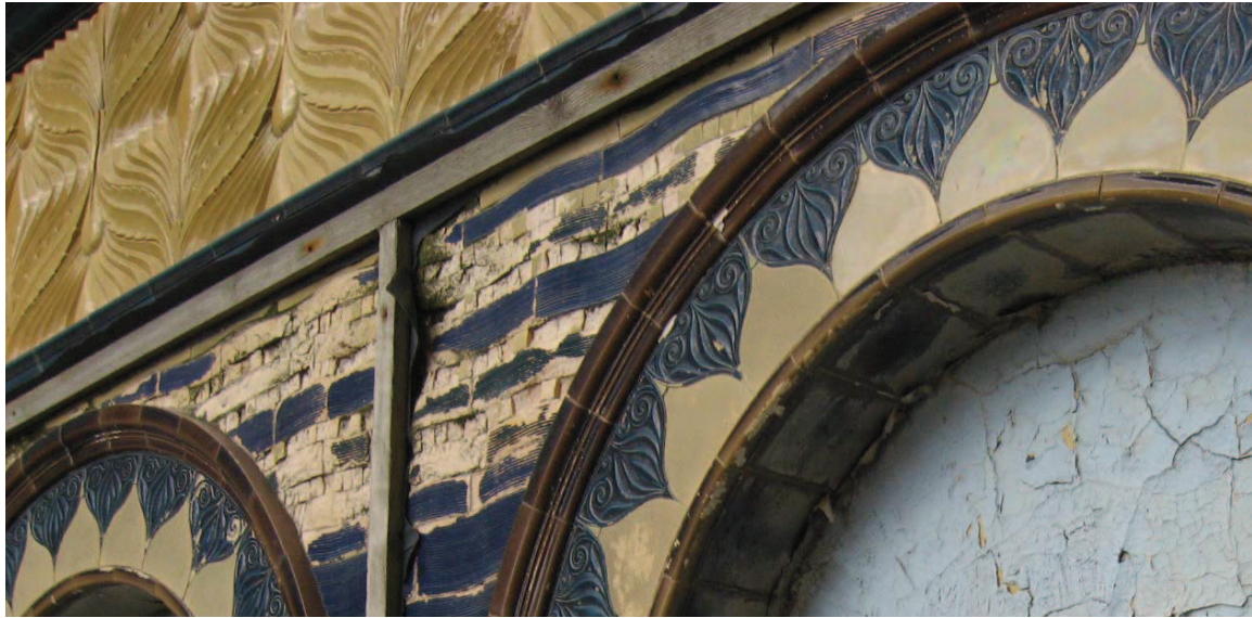
Some of the remaining original ceramic tiles used to decorate the former swimming baths at the Medina House site, Hove
